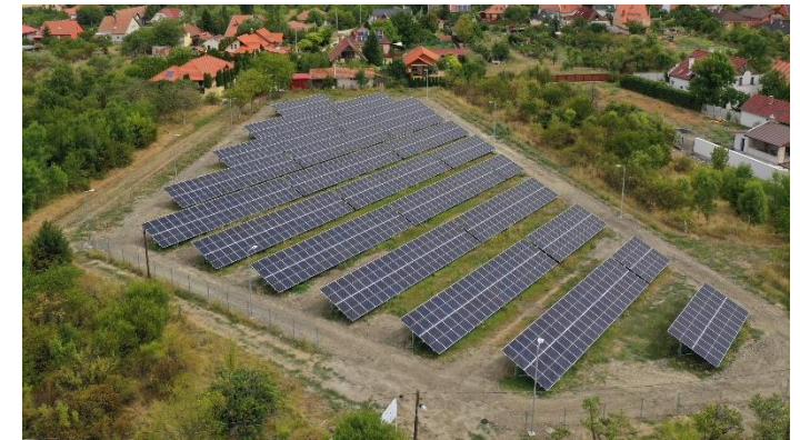
PV Park 3 331,2 kWp 828 db panel
