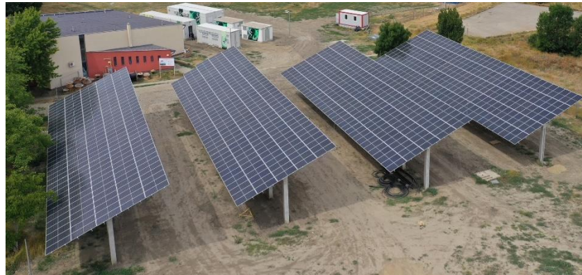
PV Park 2 281,8 kWp 702 db panel
