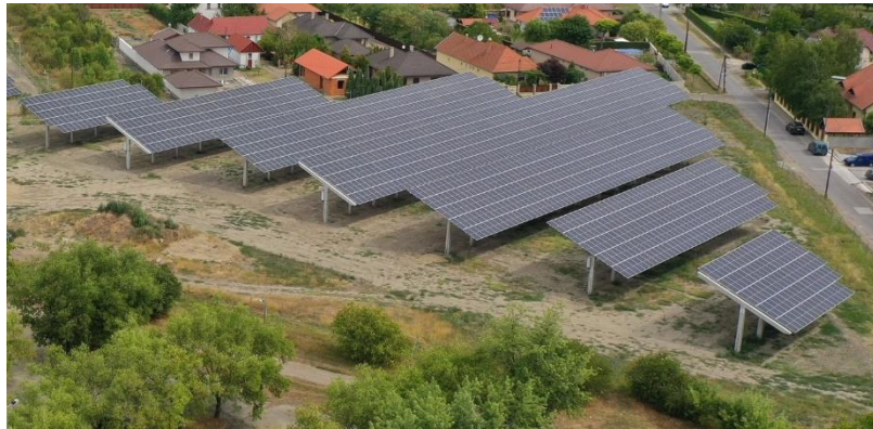
PV Park 1 684 kWp 1710 db panel
