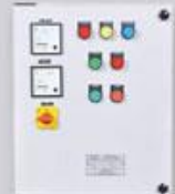
PUMP CONTROL PANEL
